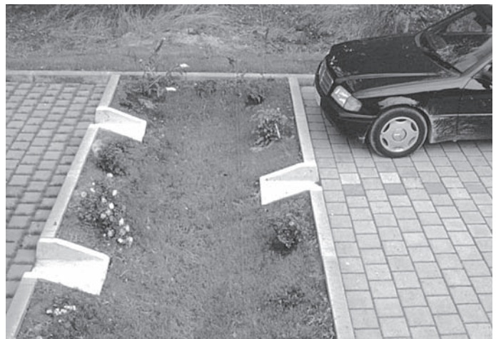
Figure 25. Curbing and drainage swale handle flows that exceed the design rainstorm.
