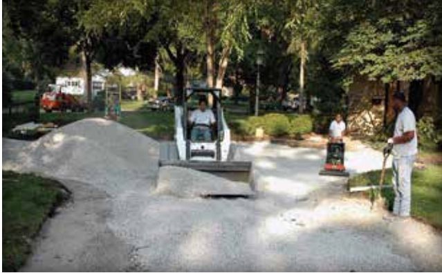
Figure 17. Perimeter berms made with dense-graded base are in place prior to placing open-graded aggregate in the driveway.
