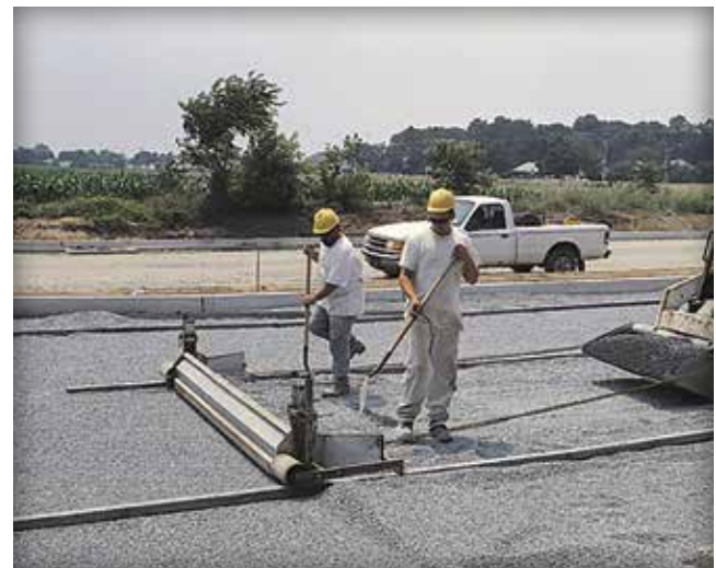
Figure 25. A screed beam pulled by equipment can be more efficient and productive.
