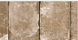
Pavers with efflorescence
